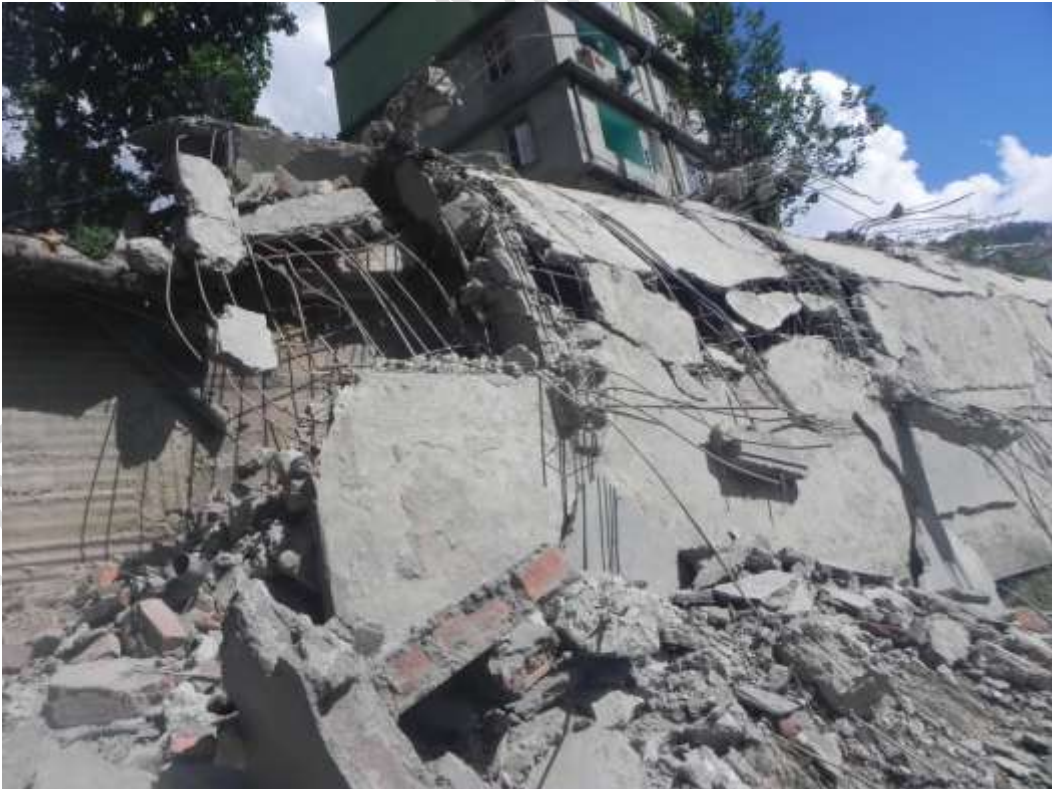
Fig: Building collapse at Gangtok due to September 18 th Earthquake
