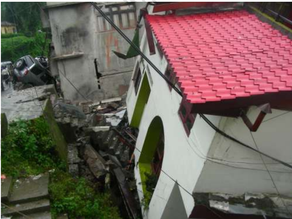
Building collapse at Balwakhani, Gangtok
