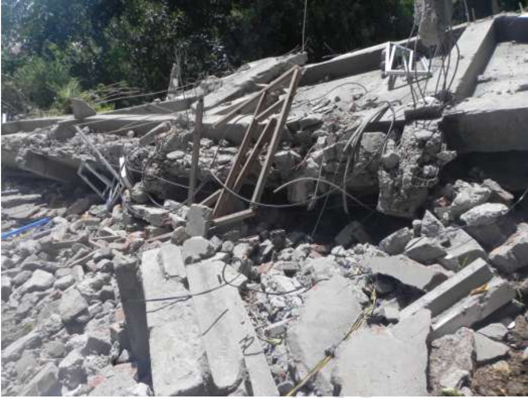
Fig: Building collapse at Lumsey, Gangtok, close view.
