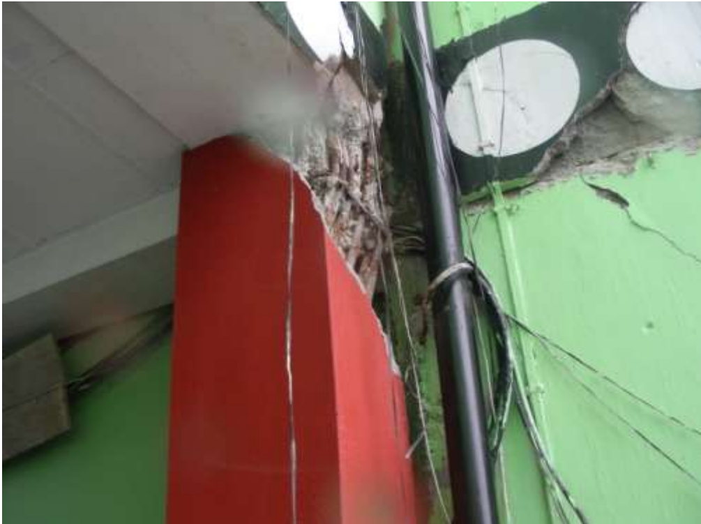
Bending of column rod at Secretariat, Gangtok
