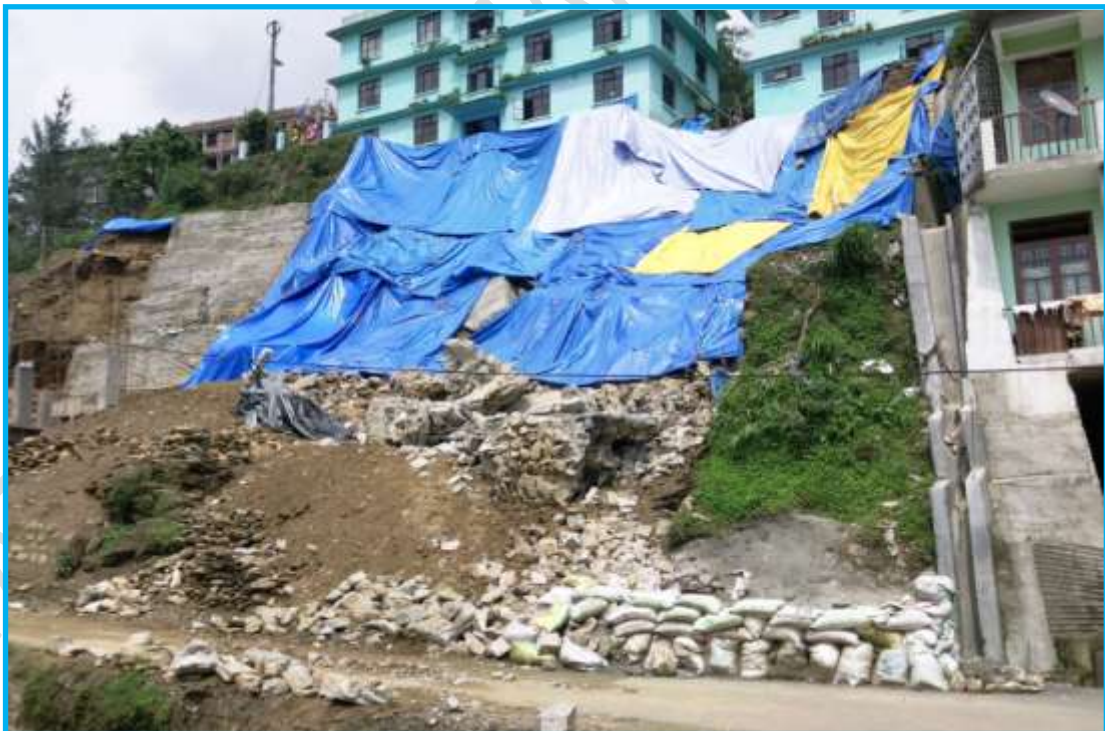
Slide at Gangtok during House Construction
